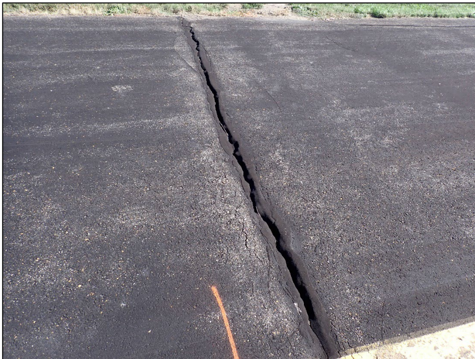
TW-01-05: L&T Cracking
