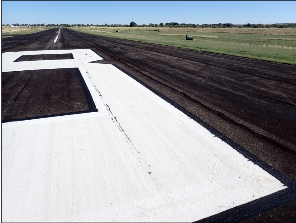
RW08-01-01: L&T Cracking
